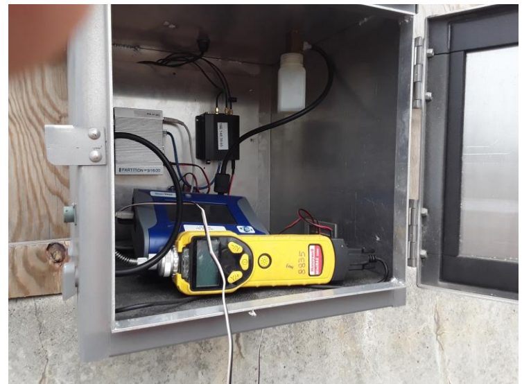
COMMUNITY AIR MONITORING STATION
