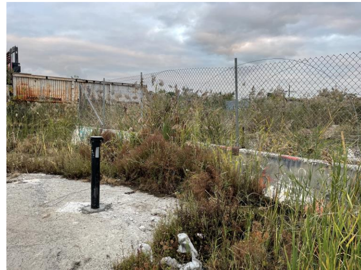
MONITORING WELL COVER
