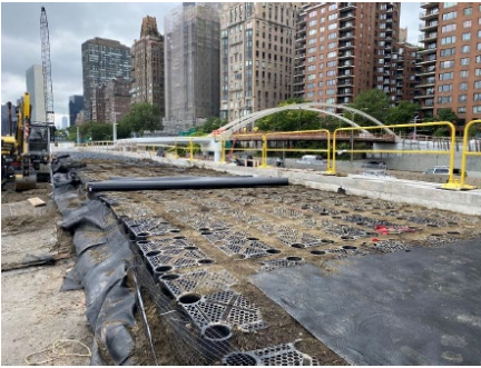
Modular pavement system installed underneath the bike path to encourage root growth by adjacent trees
